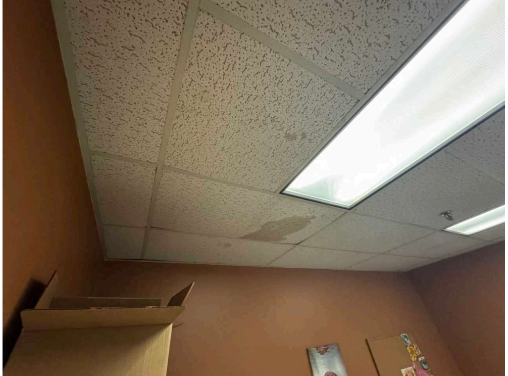
193 207-ceiling damage ground floor Date Taken: 7/10/2026
